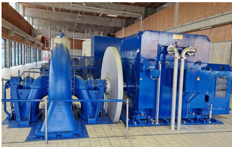
Caption: One-stop shop: Menzel built a slip-ring motor with a brush-lifting device, base frame, coupling and liquid starter, dismantled the old motor and installed and commissioned the new pump motor
